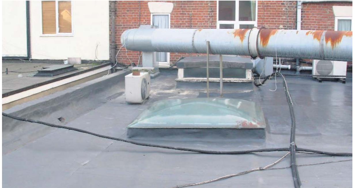
VARIED APPLICATIONS: Freedom Fibreglass Roofing utilises the latest products to provide commercial roofing systems like the one pictured above, and residential options, pictured below.
