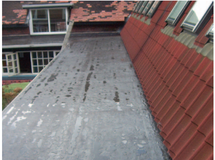
Solvent-free Kemperol was used to repair the corridor roof on this school in Lancashire without disrupting classes.
